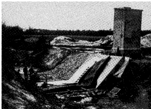
Figure 5. Reverse filter downstream of the Fabridam.
