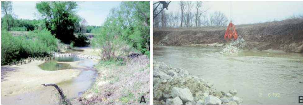
Fig. 3 Habitat rehabilitation measures in (a) Goodwin Creek and (b) Hotophia Creek. (a) Goodwin Creek reach GC_h . Existing stone erosion control spurs have been extended across the base flow channel to create a v-shaped weir. Dormant willow posts have been planted in sandy deposits downstream from weir
