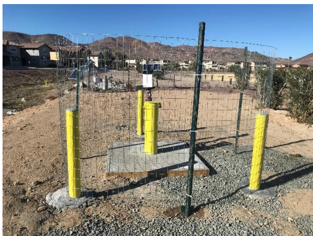
Figure 7. Completed monitoring well (MW) by GeoSystem Analysis on December 11, 2019, and data collection and maintenance by UC Riverside and USDA Riverside.
