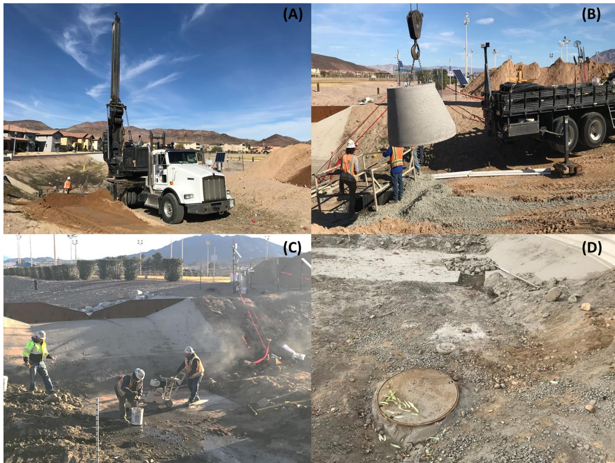
Figure 3. The installation of DW2 (A & B) and connection pipe (C) and completed well (D) at Fort Irwin on December 17 th – 21 st , 2018 by Torrent Resources, UC Riverside, and USDA Riverside.
