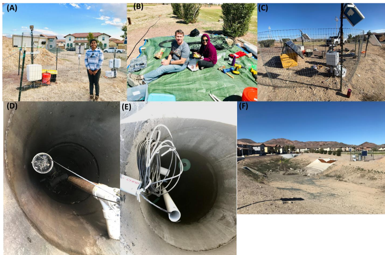
Figure 6. Installation of sensors and equipment (water level, turbidity, and remote data access) to continuously monitor the performance of drywells (A, B, & C) , the restored SC1 with a permeable net cap on overflow pipe, sensors, and connection pipe in SC1 (D) , sensors, sensor tube, piezometer tube, and connection pipes in SC2 (E) , and the complete automated operational site on April 2, 2019, monitored by UC Riverside, and USDA Riverside. All the sensors are placed at the bottom of the respective chambers, i.e., SC1, SC2, DW1, and DW2.
