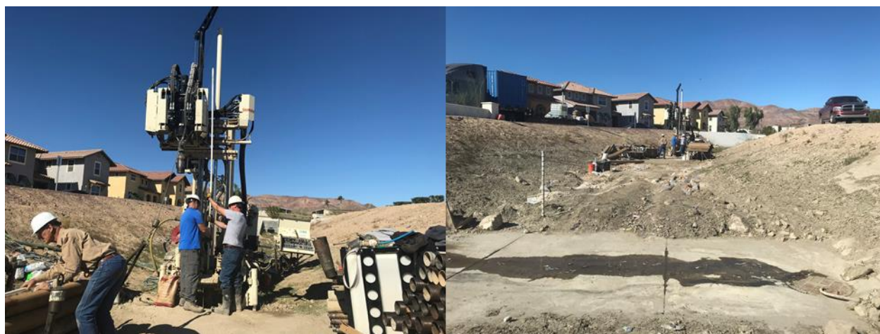
Figure 2. The installation of a test well to measure the site soil hydraulic properties on November 12, 2018, by the US EPA.
