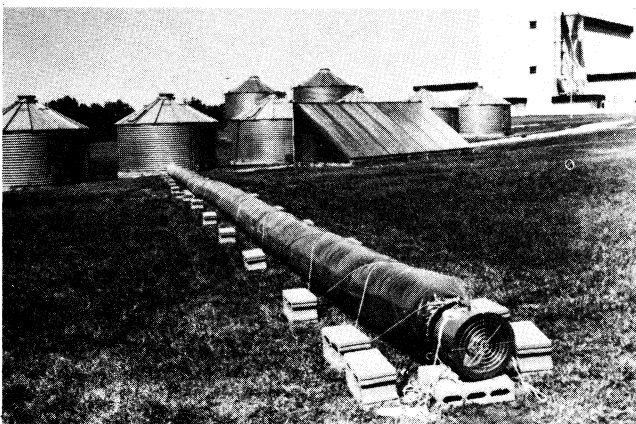
FIG. 1 Air-inflated plastic tubular solar collector used in tests 4 and 6.
