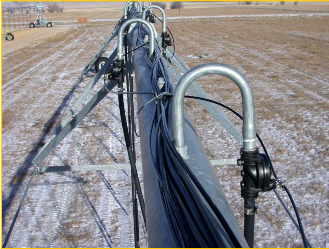
Figure 4. Valve arrangement , control wires and pneumatic tubing layout for the Nesson precision irrigation system.
