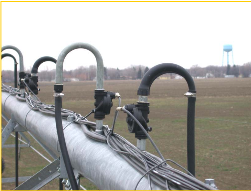
Figure 3. Valve arrangement, control wires and pneumatic tubing on the Sidney system for both the spray heads and LEPA application methods.
