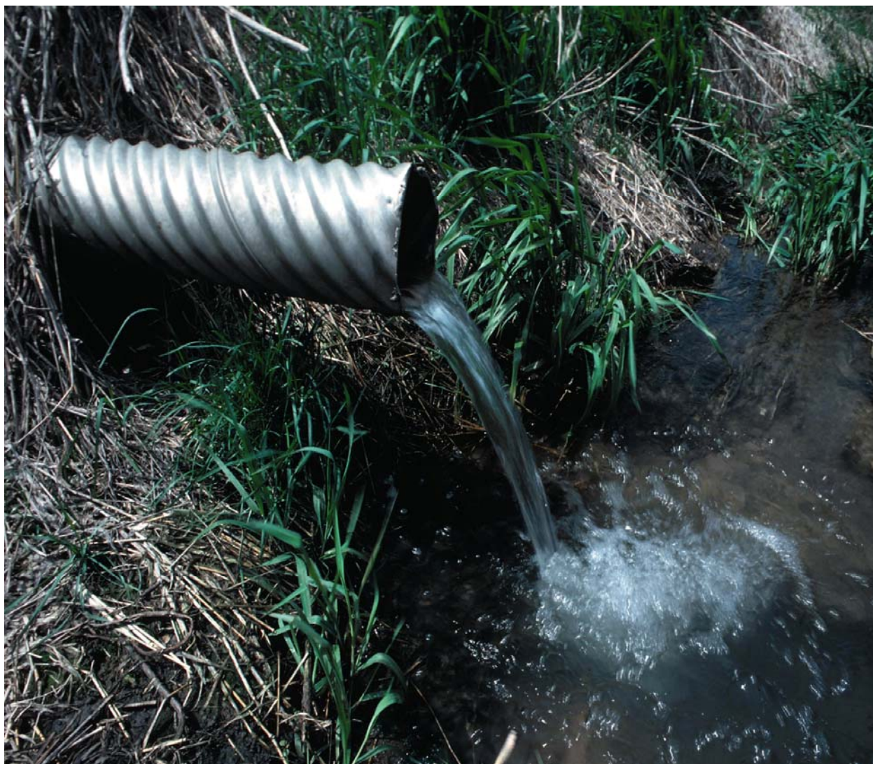
Figure V-13: Tile drain discharging into a ditch.
