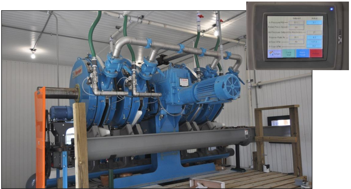
Rotary press used for solid-liquid separation. Touch-screen process control is shown in upper right photo.
