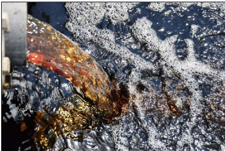
Effluent from N module into the clean water tank.
