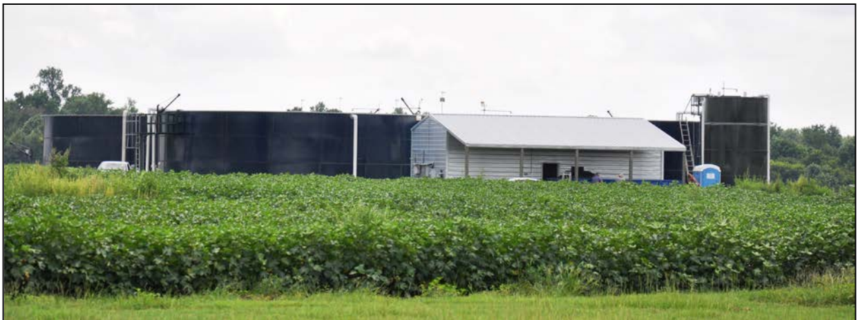
View of manure treatment system at Jernigan farm. Building contains the solid-liquid separator. Tanks at left are homogenization tank (front) and nitrification tank (back); tall tank at right is decanting tank.
