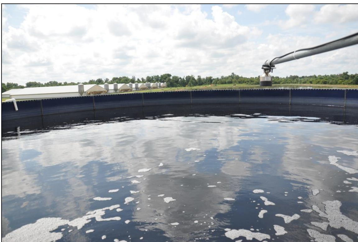
Clean water tank. It stored N treated water for recycling into the barns.
