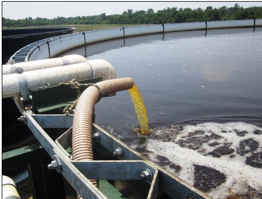
Separated manure effluent being poured into denitrification tank.
