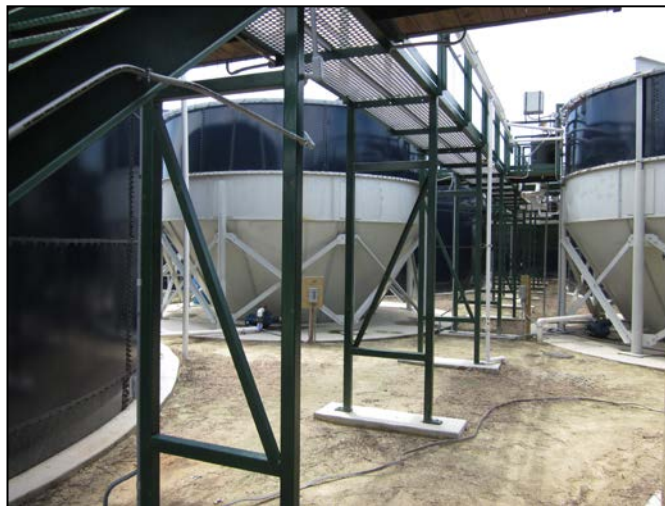
Picture shows view of plant at ground level. Cone bottom tanks are settling tanks used in nitrogen (left) and phosphorus (right) modules.
