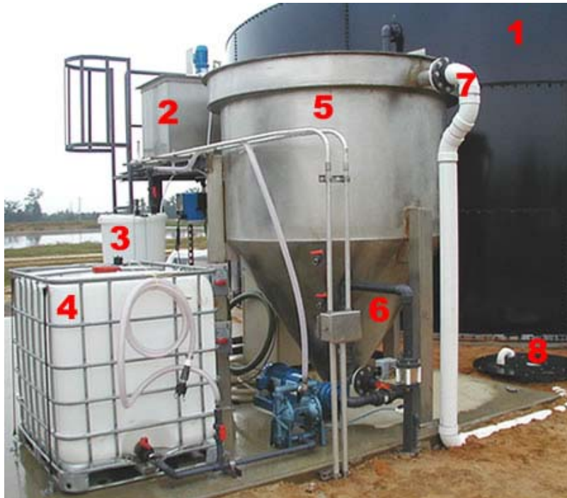
Figure 17. Phosphorus separation reactor installed at Goshen Ridge hog farm in Duplin County, NC. Storage tank (1) in background holds wastewater from which ammonia nitrogen and carbonate buffers have already been removed. This wastewater gravity flows to reaction chamber (2) along with a slurry of water and hydrated lime suspended in mixing chamber (3). More lime slurry is stored in a tote container (4) until needed. Lime slurry is 30% suspension ready to use supplied by Chemical Lime Company. Liquid flows from the reaction chamber (2) into cone-shaped settling tank (5). There, phosphorus sludge settles to the bottom (6) and is later removed, filtered, and dried in filter bags. Cleaned wastewater flows from top of settling tank via the white pipe (7) and is delivered to sump (8). An underground pipe carries cleaned wastewater to storage pond or nearby subsurface irrigation experiment for crops.
